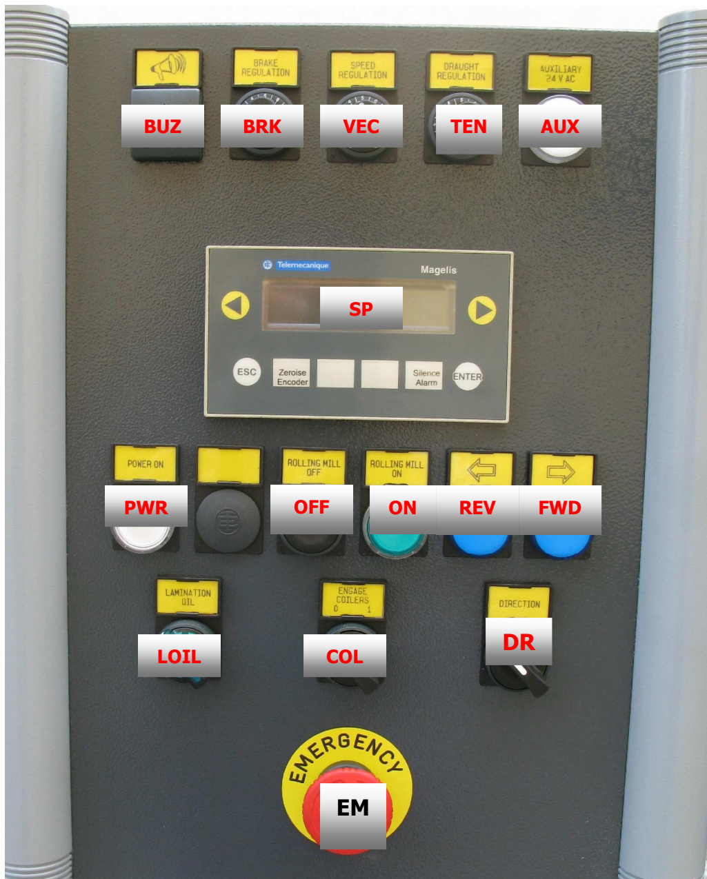
Fig. 5 – Main control Panel.
